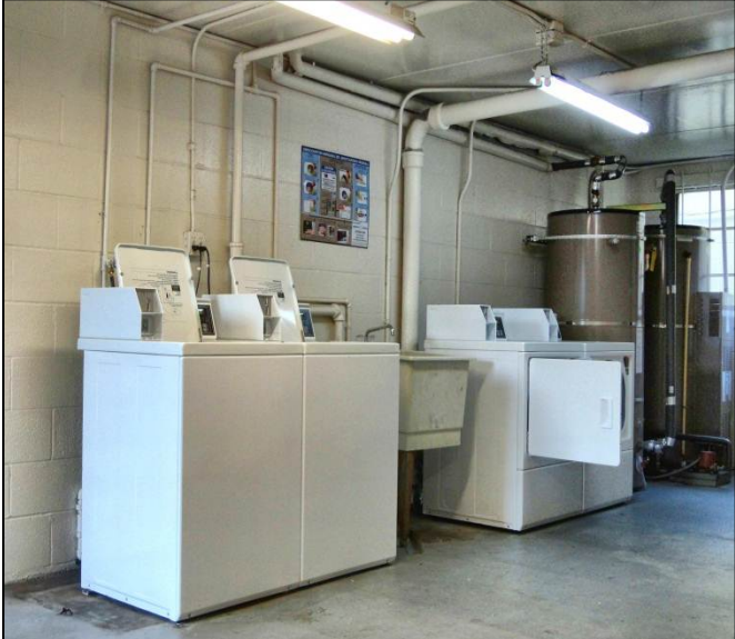
Typical Laundry Room
